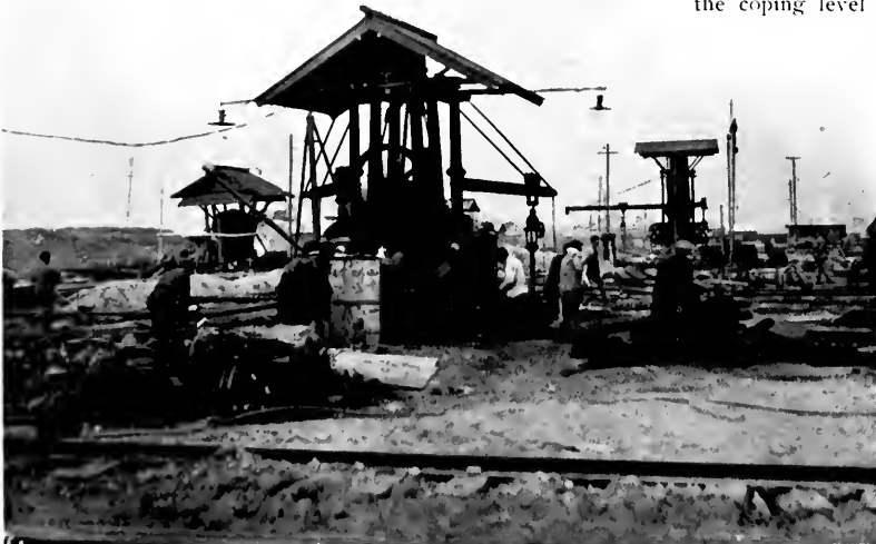
Powerful shearing machines are located at frequent intervals about the fabrication yards.
